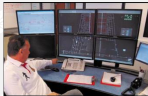
Integrated Communications & Control
